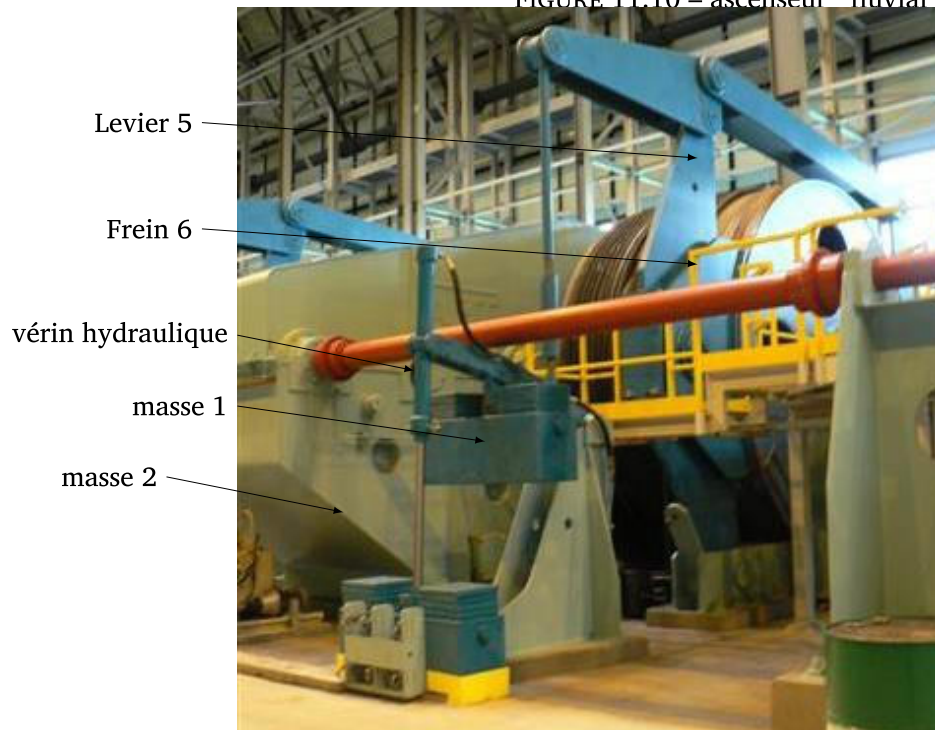
FIGURE 11.11 – salle des machine
